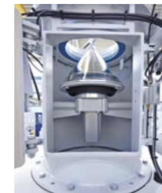
Maintenance flap at the pressure chamber
